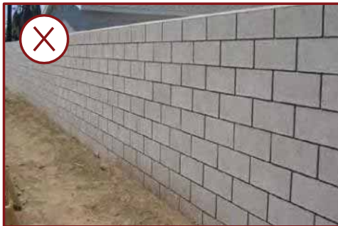
> Example of a smooth face concrete/cinderblock wall that is not permitted in the Gateway Corridor Overlay District
